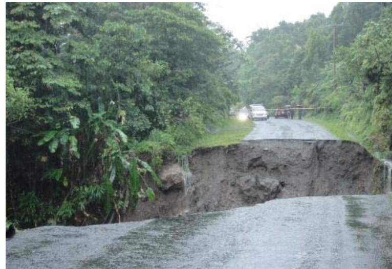
Pond Casse, Road Failure, Dominica, 2013
