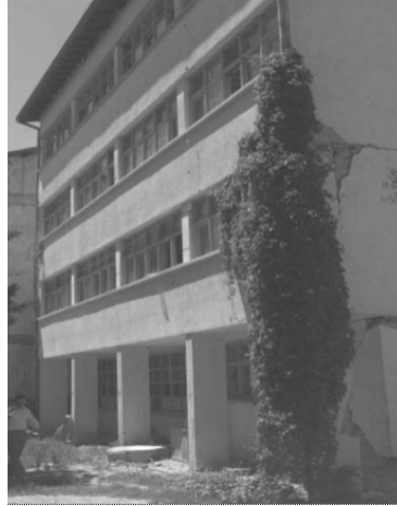
Figure 2. Digital photo in Dinar, Turkey, of the damaged schoolhouse and plumb lines used as scale information
